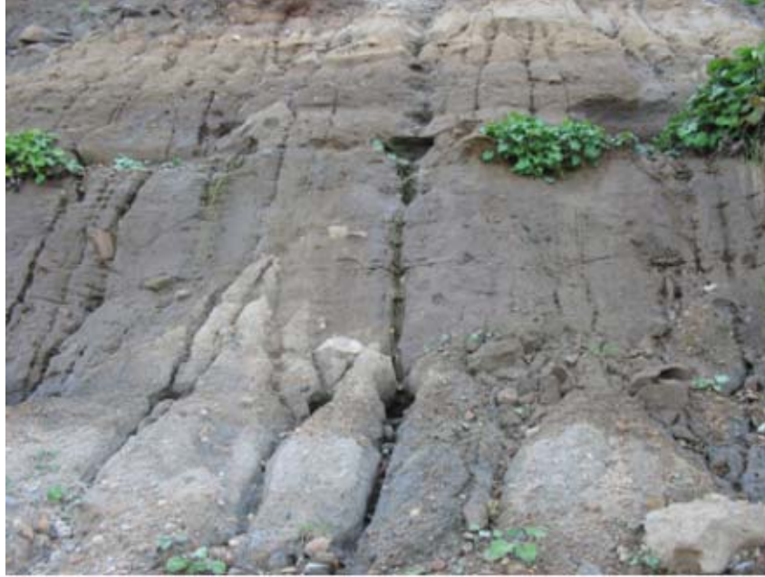
Figure 4. Groundwater seeping out of the face of the bluff where hardpan layers outcrop results in concentrated streams of water incise the face, dislodge material and undercut the clay lenses.
