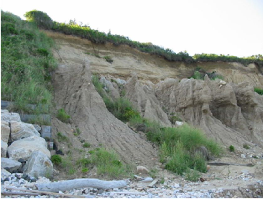
Figure 10. Bluff recession is intensified for non-stabilized regions. Erosion along the flanks of stabilized bluffs can undermine protective structures and often require periodic maintenance. Hardpan layers are visible in the photograph and long term incising of groundwater across the face has carved ridge structures, seen protruding from the face.
